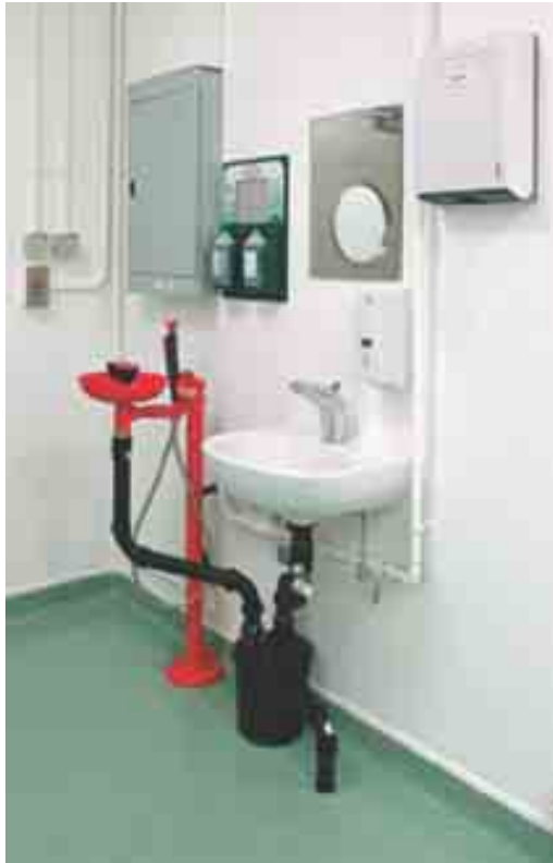
Emergency eye wash
